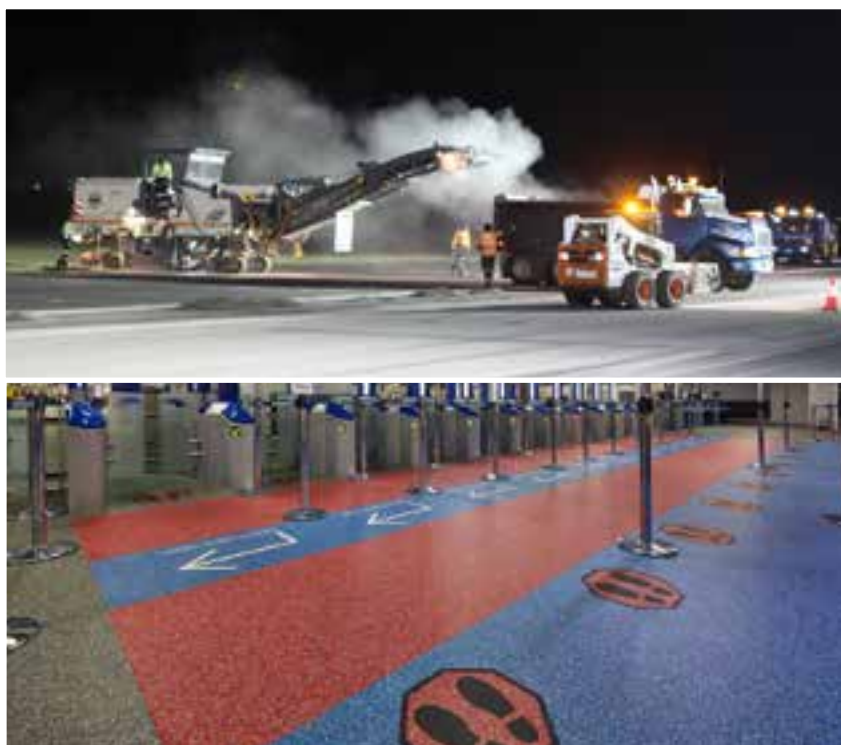
Above: 42,000 tonnes of asphalt was used in the resurfacing of BNE's main 01/19 runway Bottom: New Entry Control Point at BNE's International Terminal
